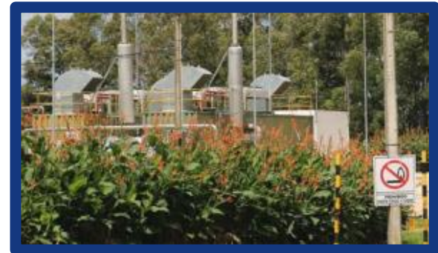
Site where biogas is converted into power, of which 25% is reinjected into the Lanús Trinidad combed wool plant and 75% is sold
